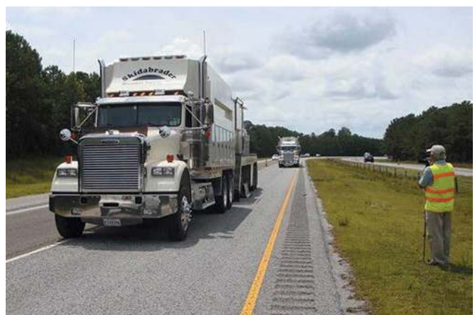
Working in tandem the two Skidabrader units, each with an effective width of six feet, covered an entire lane width in a single pass
