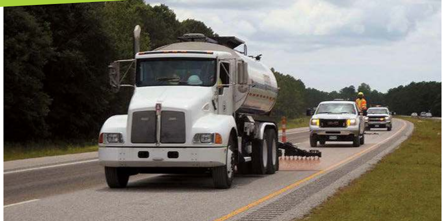
On I-40 near Wilmington, N.C., Reclamite maltene rejuvenator is applied with a Bear Cat computer-controlled 2,500 gal distributor truck
